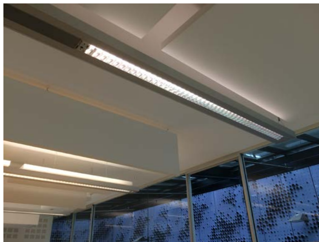
Figure 19 – Lamps in an intelligent building
