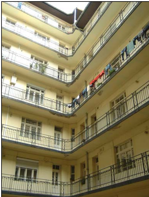
Photo 7.3 Hanging corridors in the inner courtyard of a tenement block built at the beginning of the 20th century
