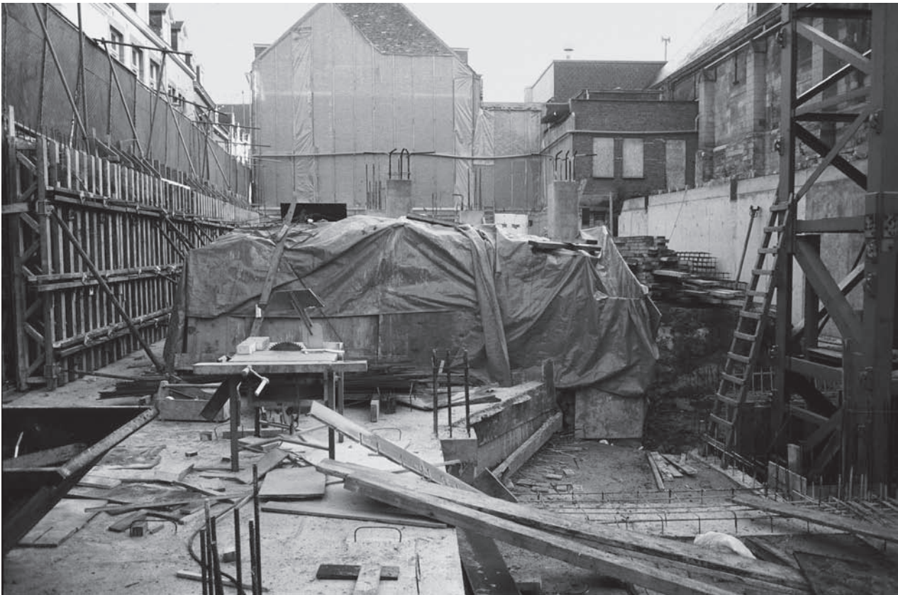
Fig. 3. The Hotel Derlon site during building activities in the winter of 1983–84. In the centre, the fortress wall has been protected by wooden boarding and plastic tarpaulin.
