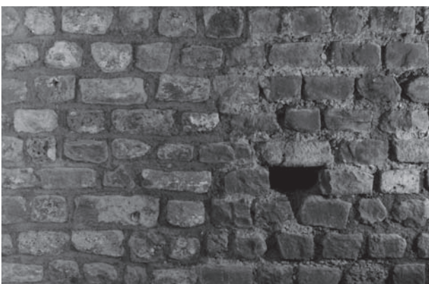
Fig. 8. Detail of the masonry of the late-Roman west wall at the inner side: on the right can be seen the consolidated original joints, on the left the renewed joints where the mortar has been pushed back a little bit.
