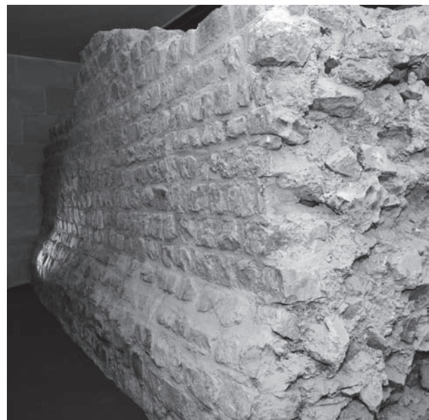
Fig. 9. The exterior of the west wall (land side) was only displayed after the 2007 renovations. Most of the joints have been renewed.
