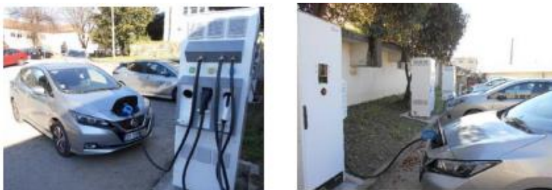
Fig. 2. Electric vehicle charging stations.
