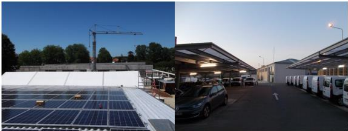
Fig. 3. Overview of the implemented PV plant.
