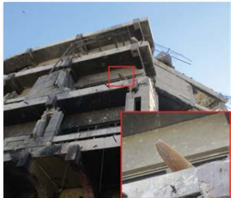
Image 6. A 500 lb. bomb located on the fourth floor of a building with the stairs mostly destroyed, West Mosul, Iraq.
