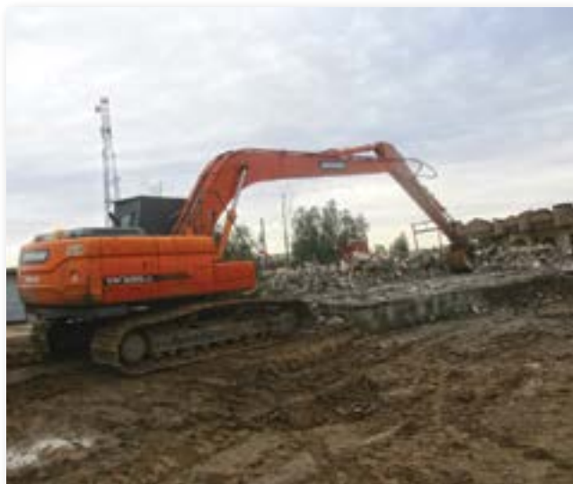
Armored excavator from FSD’s mechanical clearance team in Iraq removing rubble so that villagers can return to their land and rebuild their homes and livelihoods. Image courtesy of FSD.
