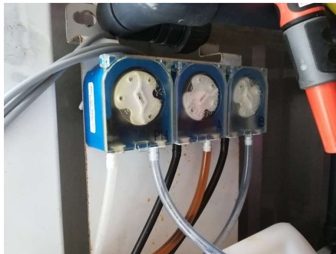
Figure 18 - Peristaltic pumps used to mix nutrients and acid into the main tank
