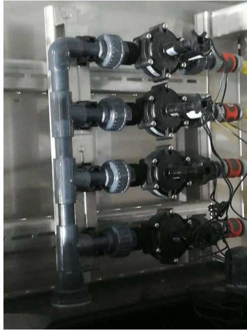
Figure 19 - Automatic Valves for the gully rack
