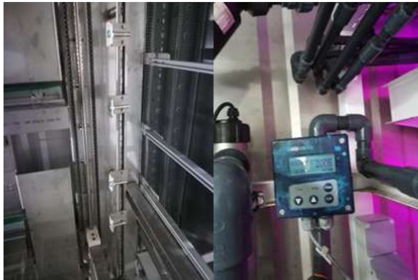
Figure 11 - On the left: Elevator Sensors; On the Right: EC Sensor
