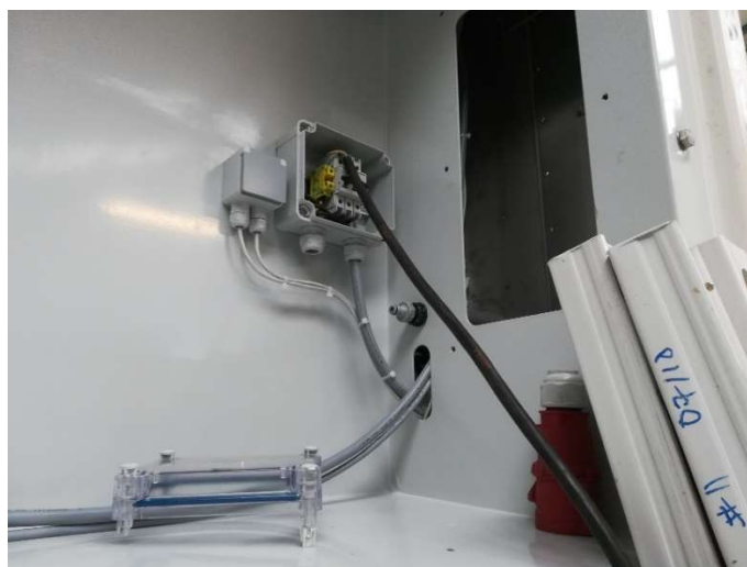
Figure 22 - Connections for the AC unit, electricity and water intake
