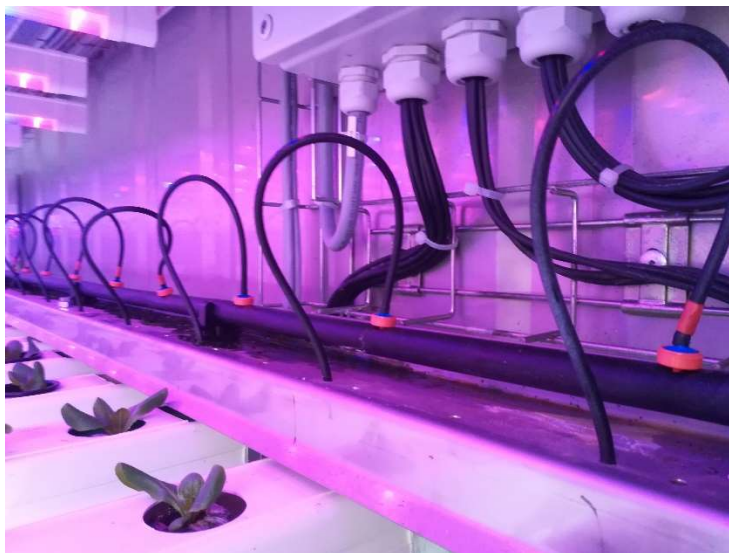
Figure 20 - Close-up of the flow limiters installed on the drippers
