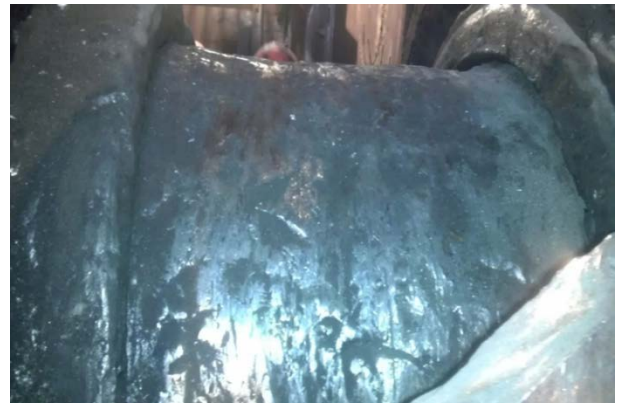
Figure 2. Surface of the trunnion of the converter support ring after the destruction of the bearing.
