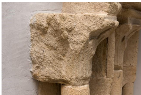
Fig. 4. Damages of the stone column capital
