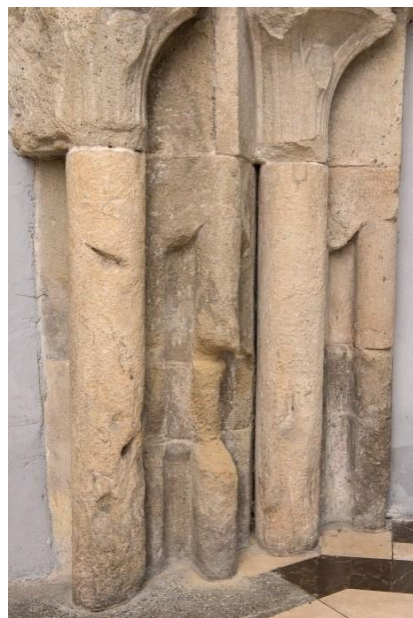
Fig. 3. A section of the portal, with visible damage of the elements of the portal jamb. Condition before the removal of the bottom parts
