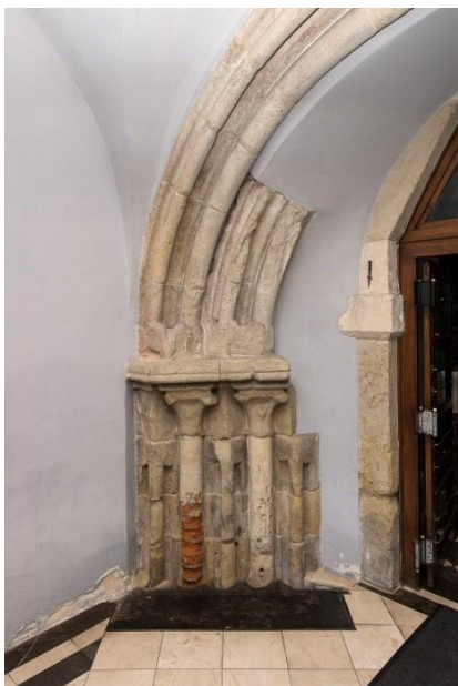
Fig. 2. A section of the portal, with visible decay of the material and the brick infill replacing a section of the former column. Condition before the removal of the bottom parts
