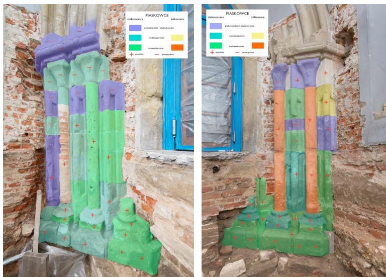
Fig. 7. Breakdown of the sandstones used for the jambs of the portal according to their colour, grain, and presence of calcium carbonate
