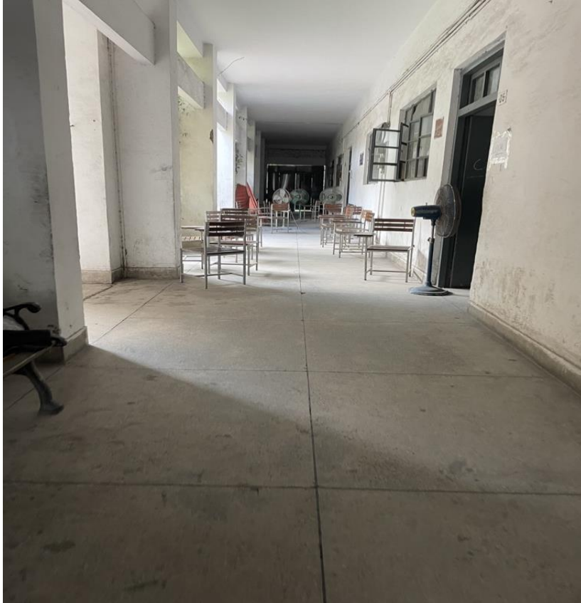
Figure 8: Corridors of Dharampura College where chairs and pedestal fans are dragged in the corridor for young women to sit and chat.
