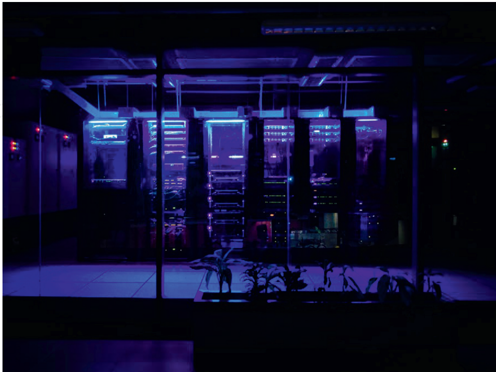
Figure 1. APU data centre.
