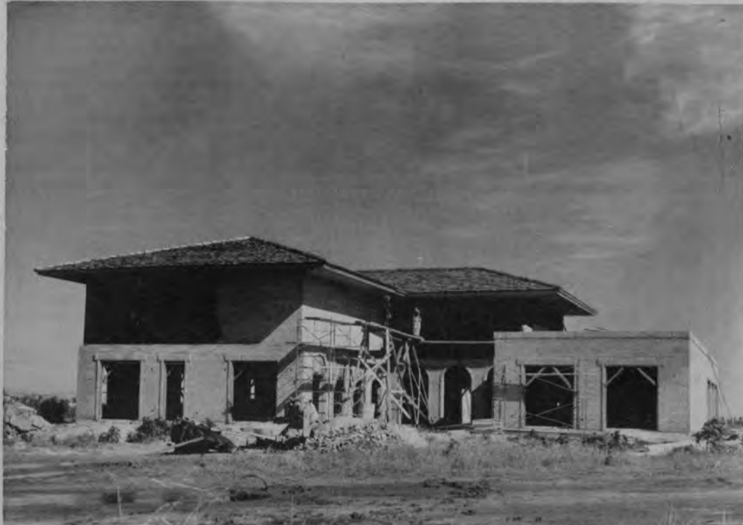
NEW HOME FOR PAN AM PRESIDENT--work is progressing on the new two-story home in Edinburg to be occupied by the Pan American College president, Dr. Ralph Schilling. Architect for the project estimates the house will be completed in April. When finished, the home will contain approximately 5,000 square feet with the first floor reserved for college activities and the upstairs assigned to Dr. and Mrs. Schilling. The Spanish designed home is located on a five-acre tract on Sugar Road, about a mile south of the Pan Am campus.
