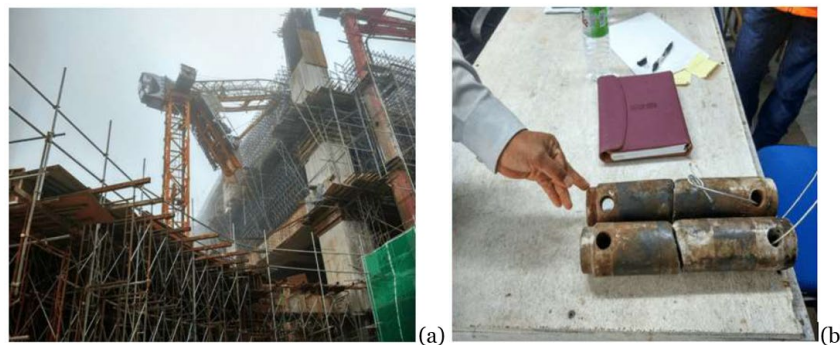
Figure 3. Tower crane accident – (a) crane after accident, and (b) broken pins
