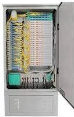
Gambar 6 Optical Distribution Cabinet
