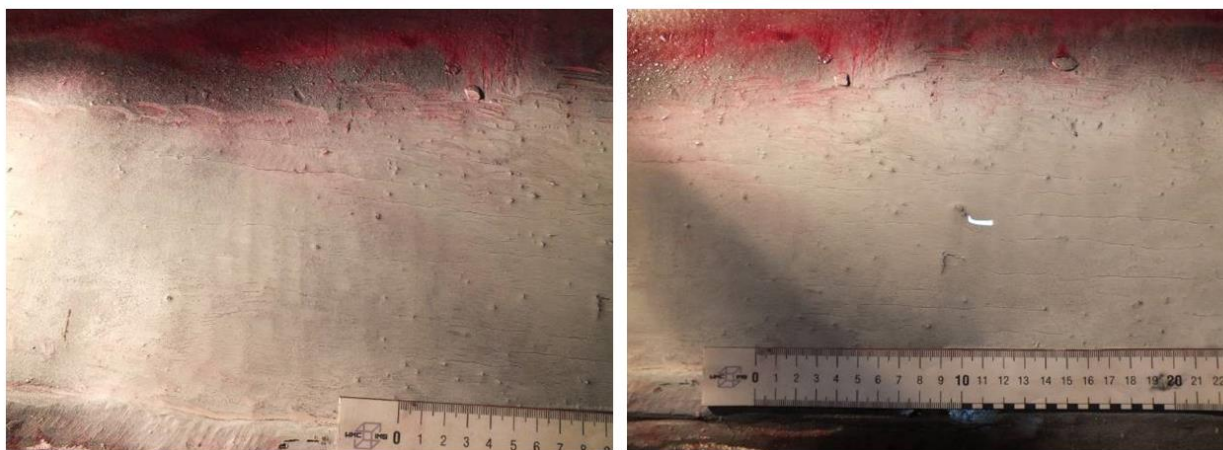
a) Appearance of the crack at the surface of the heat-affected zone
