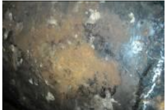
b) Pitting corrosion at the surface – VT
