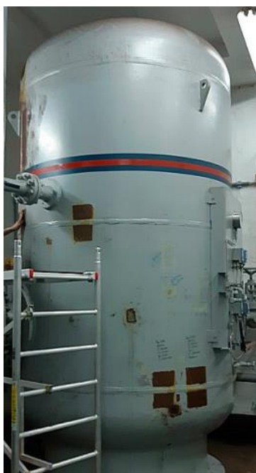
Figure 1. The pressure vessel 970, before repair.
