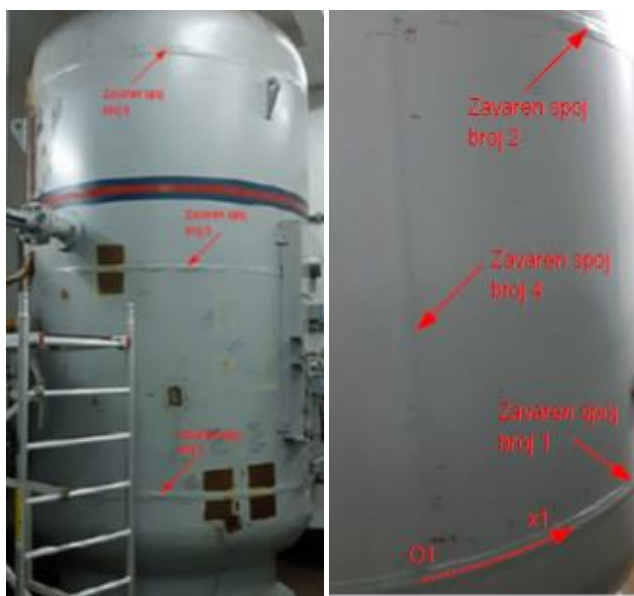
Figure 3. Tested welded joints (marked by red arrows) on vessel 970, before repair.
