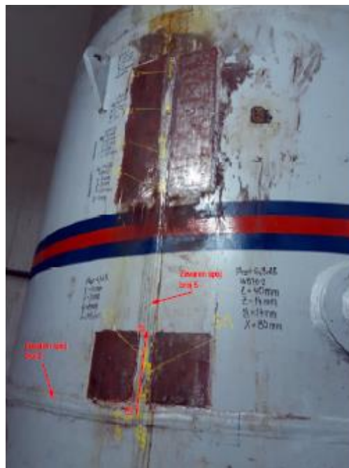
Figure 4. Tested welded joint 5 on vessel 970, before repair.
