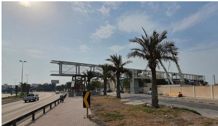
Figure 4.36: The under-construction pedestrian bridge connecting Bu Maher Fort and the Pearling trail
