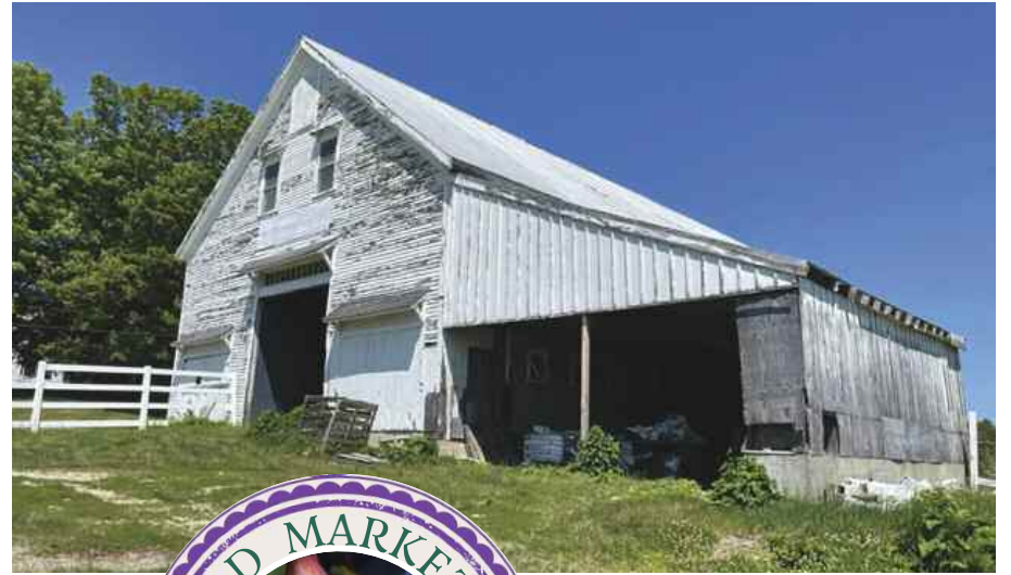
The barn at Hurricane Valley Farm is in need of restoration
