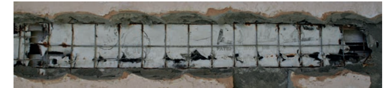
Fig. 22: Detail of damage to Stucco and STEELTEX Wire Lath
