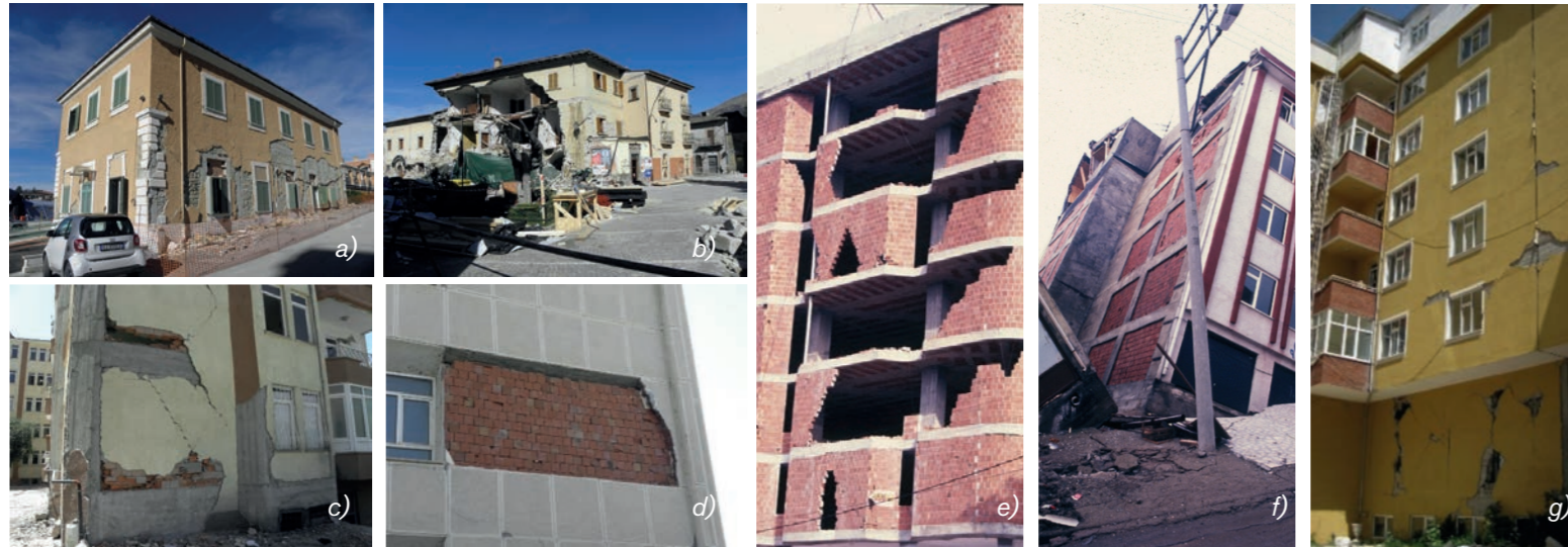
Fig. 5. Various types of seismic damages to building structures: a) Nonstructural damage to a RC building in the 2016 Amatrice, Italy EQ b) Partial collapse of a masonry building in the 2016 Amatrice, Italy EQ c) Exterior nonstructural wall damage in RC building in the 2011 Van, Turkey EQ d) Brick sandwich wall failure in the 2011 Van, Turkey EQ e) Out-of-plane failure of exterior walls in the 1999 Kocaeli, Turkey EQ f) RC building failure from soil liquefaction in the 1999 Kocaeli, Turkey EQ (no damage to nonstructural members) g) Exterior nonstructural wall damage in RC building in the 2011 Van, Turkey EQ.
