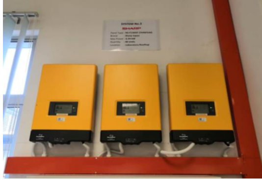
Figure 1. UTeM solar PV system
