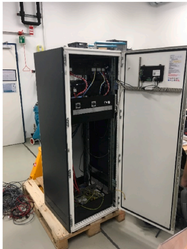
Fig. 3. Photo of the measured HSS – battery modules already disassembled.
