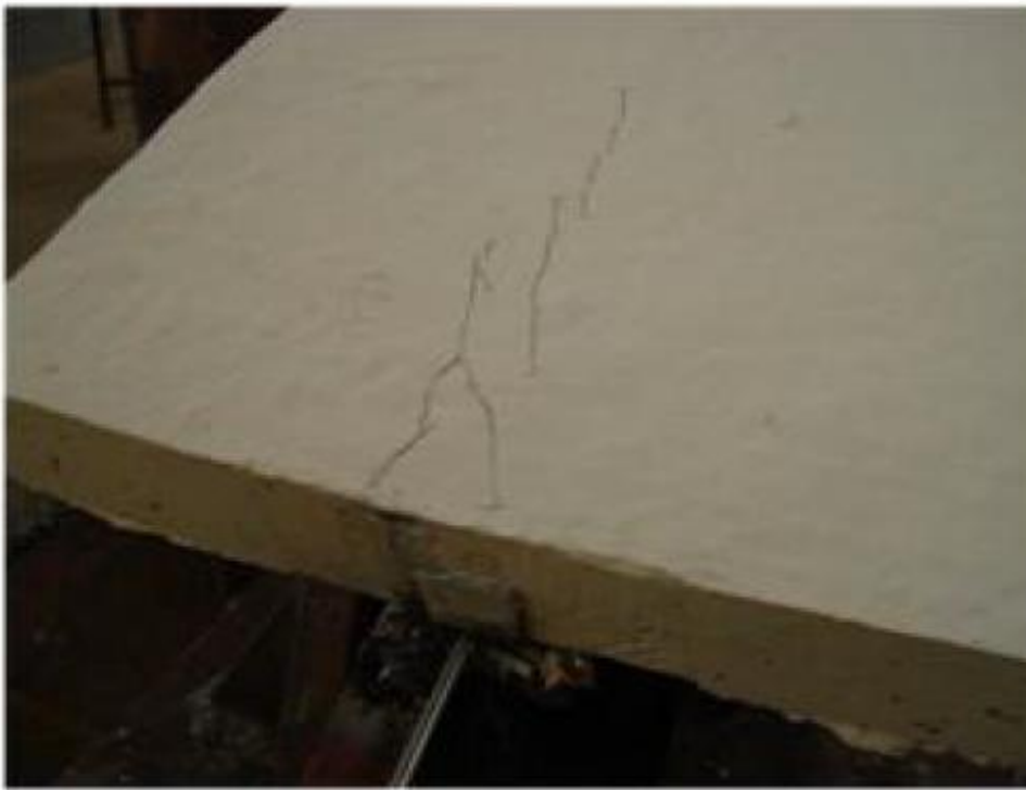
(b) longitudinal crack at the right end (Husain et al., 2013)
