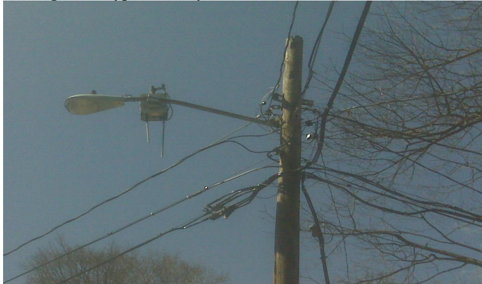
Figure 3. Typical Utility-Pole-Mounted Network Node
