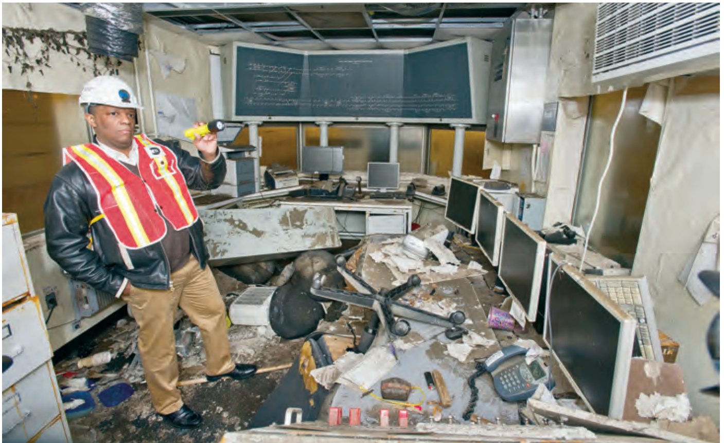
Damage to South Ferry 1 subway station in New York City after Superstorm Sandy.
