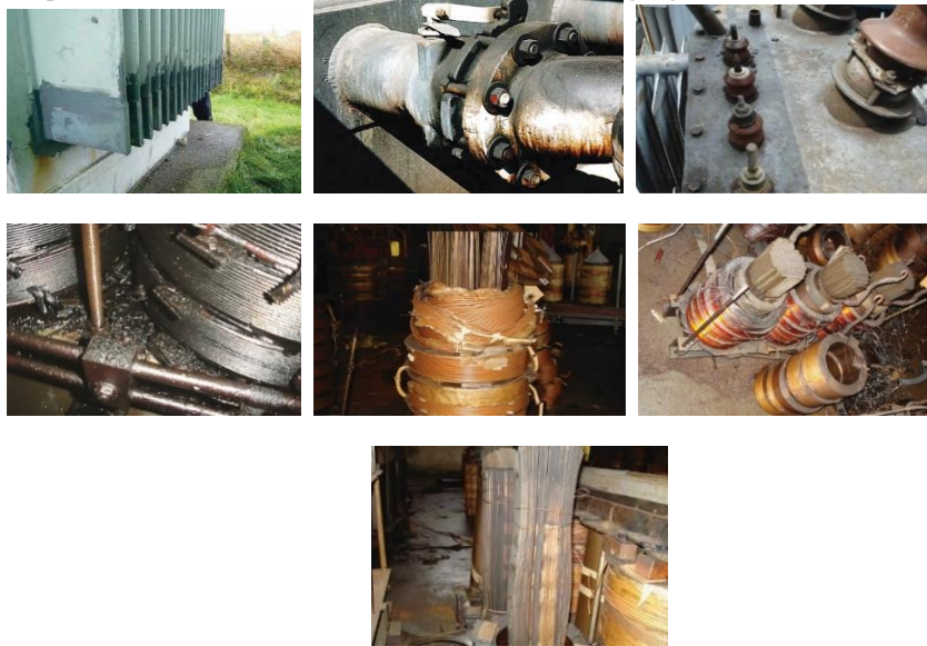
Fig. 3. Failures in the power transformer: (a) Oil leak from the radiator and (b) gaskets; (c) Released connections; (d) Moisture damage to transformer oil; (e) Strengthening the coils; (f) failure due to shrinkage and (g) Failures from magnetic circuit insulation
