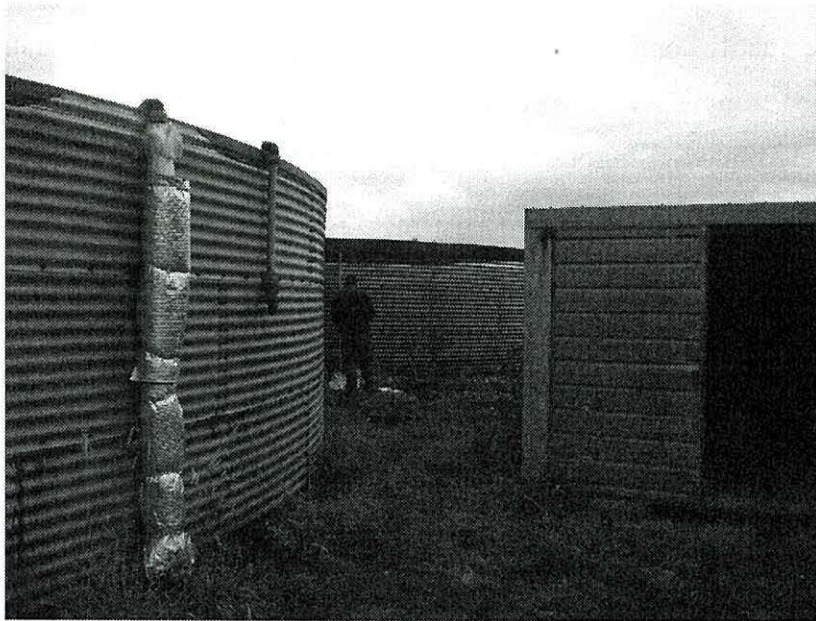
Figure 9.8: The water tanks that are filled using the Ness Gardens Borehole. The water is used to water the plants in the botanical gardens.
