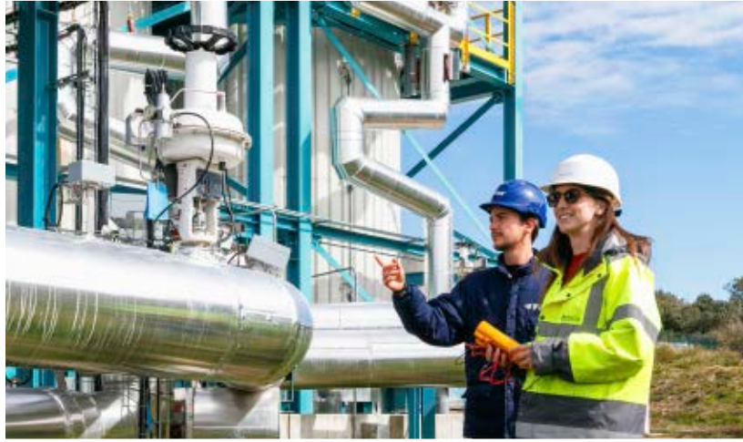
Personnel from the University of Évora and TSK Flagsol check part of the plant
