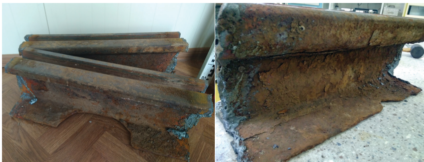
Figure 2. Rail degradation noticed at urban tracks
