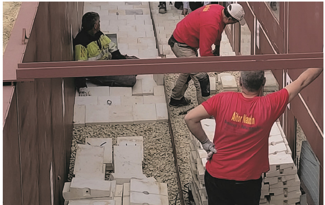
Figure 6. Picture of the placement of the WSB on the gravel bedding layer.
