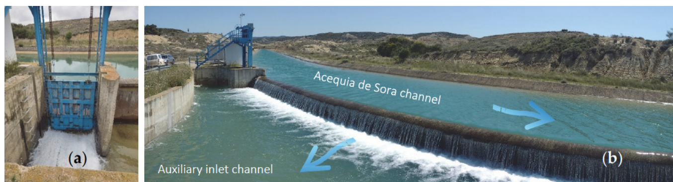
Figure 2. Intake work in the Acequia de Sora channel: (a) View from downstream of the flow control gate in operation. (b) Flow control structure on the left and side spillway from the Acequia de Sora to the auxiliary channel.
