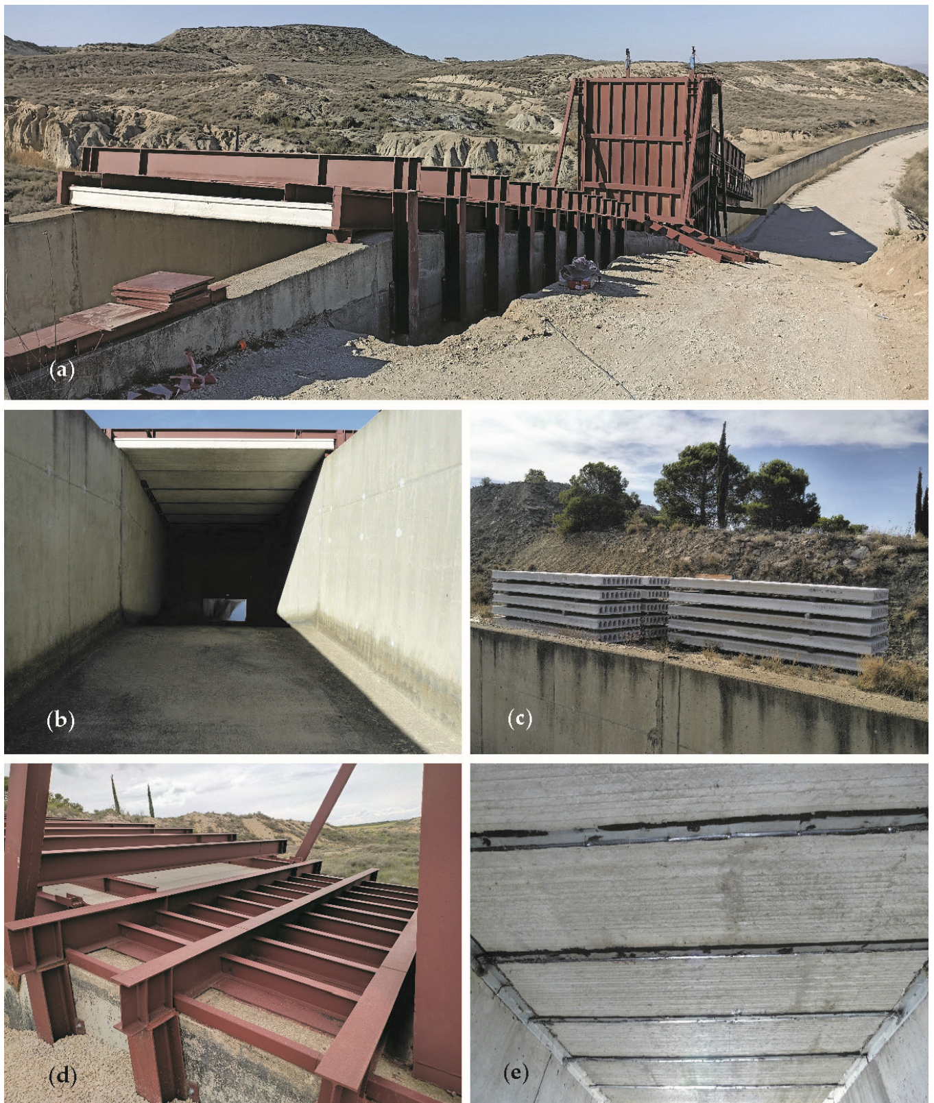
Figure 4. (a) View of HEFLR from the right bank of the auxiliary channel. (b) View of the interior of the auxiliary channel from upstream of the pressure channel. (c) Storage of the honeycomb slabs used to cover the pressure channel. (d) Metallic frames used to support the honeycomb slabs of the pressure channel and the metallic plates on the connection to the tower supply. (e) Detail of the sealing between the slabs and the channel walls (view from inside the pressure channel).
