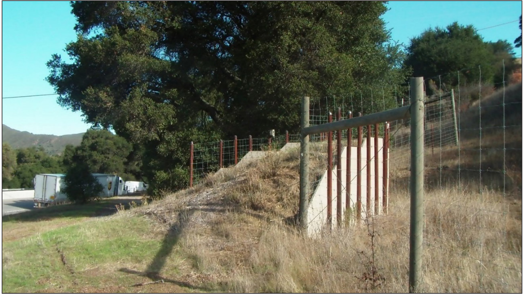
Figure 1. Jumpout ramp C (TjCK-N) along Highway 101 in San Luis Obispo County, California, USA (photo courtesy of the authors).
