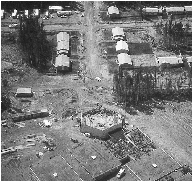
1968. Building the Mackenzie Elementary school, an Allan Greenwell plan - notice the hexagonal gym. Photo courtesy of Mackenzie and District Museum
