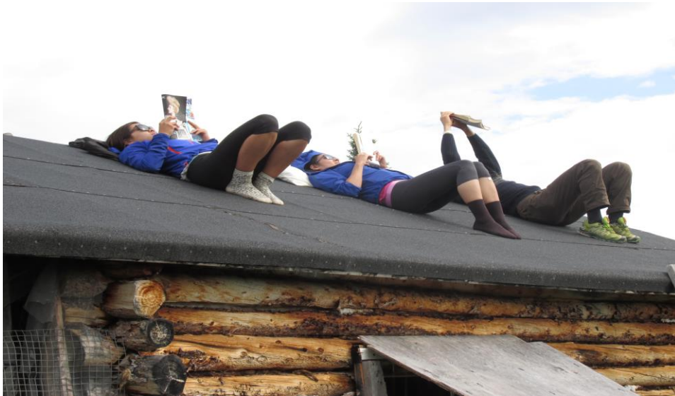
Briana, Ashlyn and Graeme busy repairing the roof of the old Schaeffer Cabin; base camp of the core study area.
