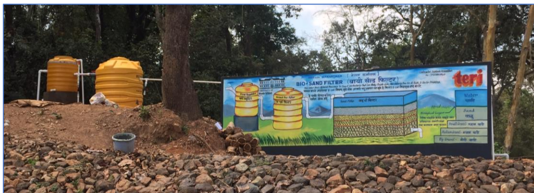
Figure 3. Picture of the IBF filter system. A diagram was painted on the filter wall giving a simple explanation of the system in both English and Marathi, the local language.
