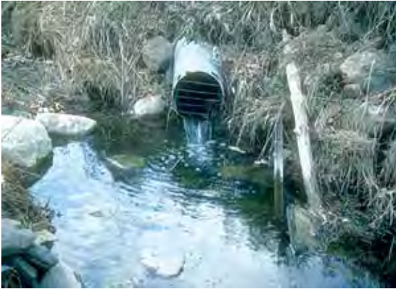
Figure 17.20. A subsurface drain line discharges into an edge-of-field ditch, diverting groundwater to surface waters.
