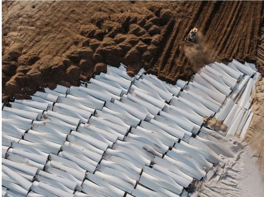
Figure 5.4: Aerial imagery of a wind turbine landfill being covered by dirt via a bulldozer. (Source: Bloomberg)
