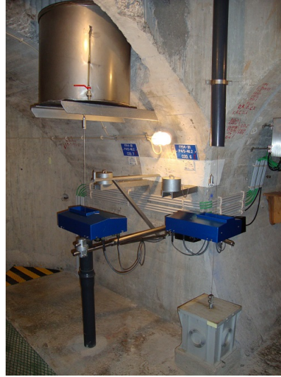
Fig. 1.15: Pendulum, measuring table and automated system for horizontal displacement measurements.
