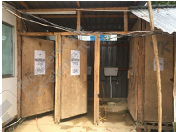
Fig. 7 Construction site C workers' quarters' utility cables hanging lowly across the quarters
