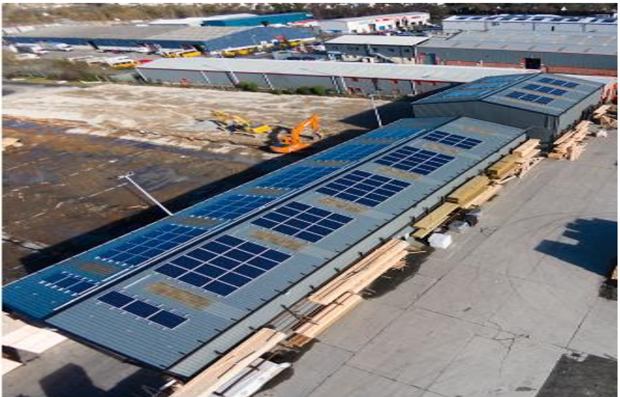
Figure 35. Examined PV arrays installed at Newry
