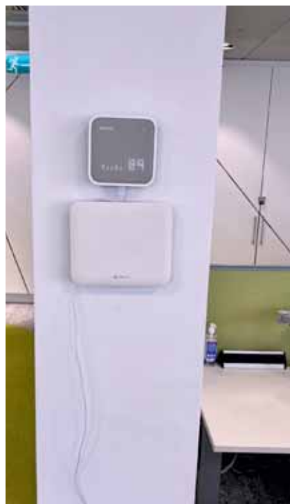
Fourth floor Kaiterra sensor.
