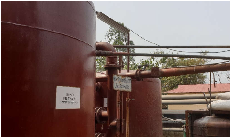
Figure 10.8 Water treatment plant in one of the case study units Source: Author (2020) in field visit of case study units
