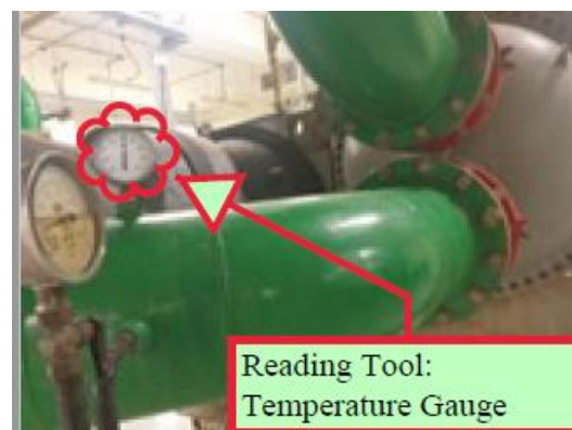
Figure 5. Cooling Tower Reading Tool.
