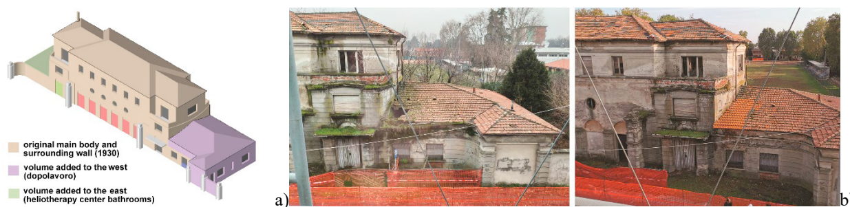
Fig. 2. Palazzo Littorio of Caronno P.: a) a schematic axonometric view of the three volumes; b) Roof photo of the north side towards the west corner before (left) and after (right) the urgent repair works in 2020. 3-types of tiles are easily recognizable: the oldest dark ones, the newest brilliant red ones and the other most diffused dull red ones.
