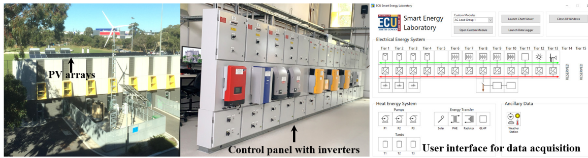
Fig. 15. PV system facility installed at Edith Cowan University.
