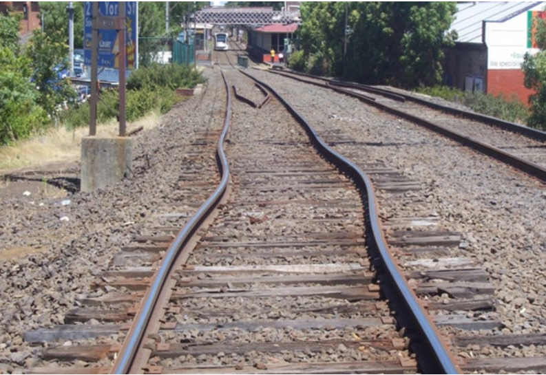
FIGURE 3: Rail buckling due to high ambient temperatures
