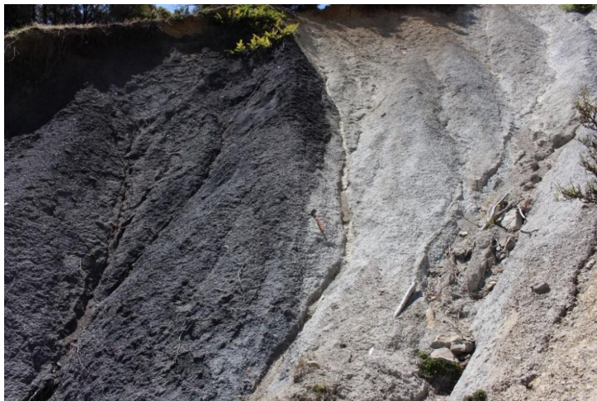
Figure 3-11. Zoom of rectangular area of Fig. 3-4f. The crushed zone consists of dark grey coloured sheared argillite and light grey coloured crushed sandstone in the Blackley area. A Niwashi in the centre of the photo shows the scale. The boundary between the two types of rocks is sub vertical.
