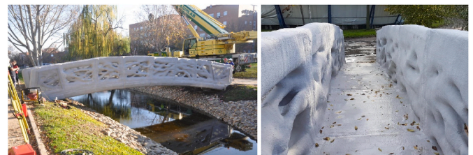
Fig. 5. a) Support and leveling operations of the footbridge and b) walking area of the deck.
