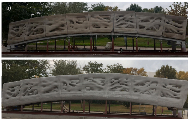
Fig. 4. a) Segments supported onto the arched steel frame and b) painted footbridge with the steel frame already embedded.
