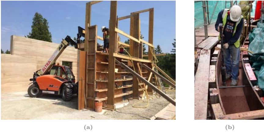
Figure 2.9: Modern rammed earth building technique: (a) construction site (©Aerecura Rammed Earth Builders) and (b) compaction with pneumatic rammer (©Rammed Earth Consulting).
