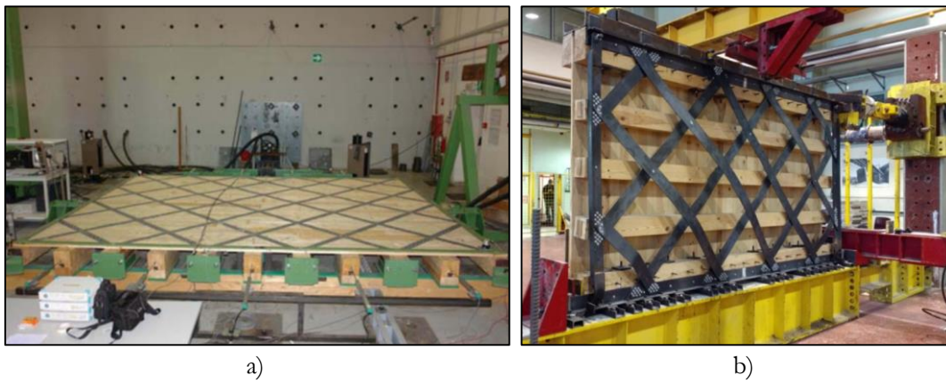
Figure 2.37 Seismic retrofitting of timber slab a) steel strips at top, b) steel strips at bottom [124]
