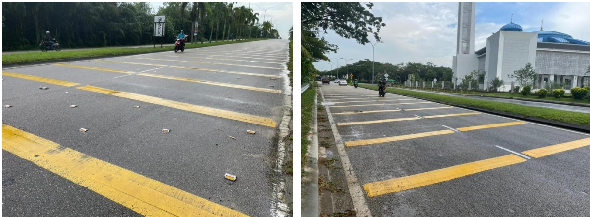
(a) TRS with road studs
