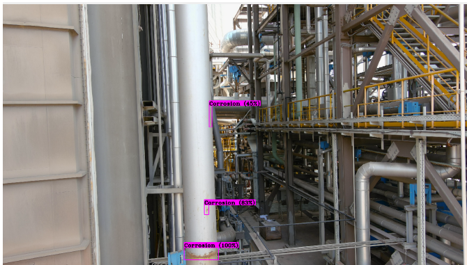
Fig. 5. Corroded areas on critical infrastructure.
